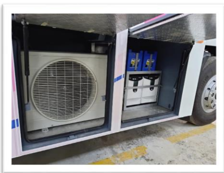
Power inverters and AC Unit
