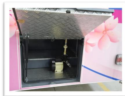
Water pump for the overhead water tank
