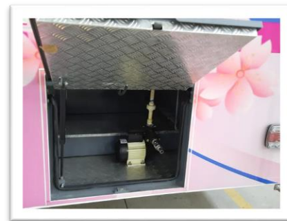
Water pump for the overhead water tank
