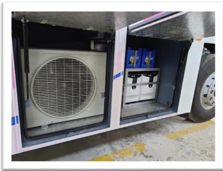
Power inverters and AC Unit
