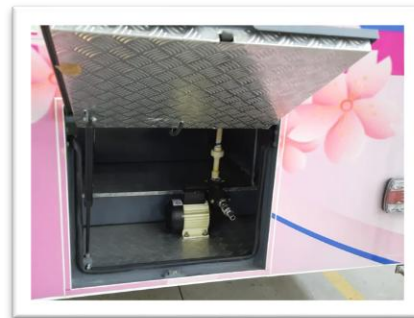
Water pump for the overhead water tank
